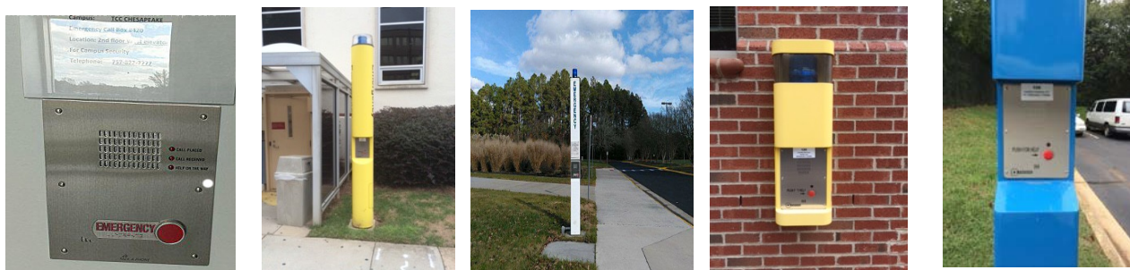
Figure 1. Emergency Call Boxes
